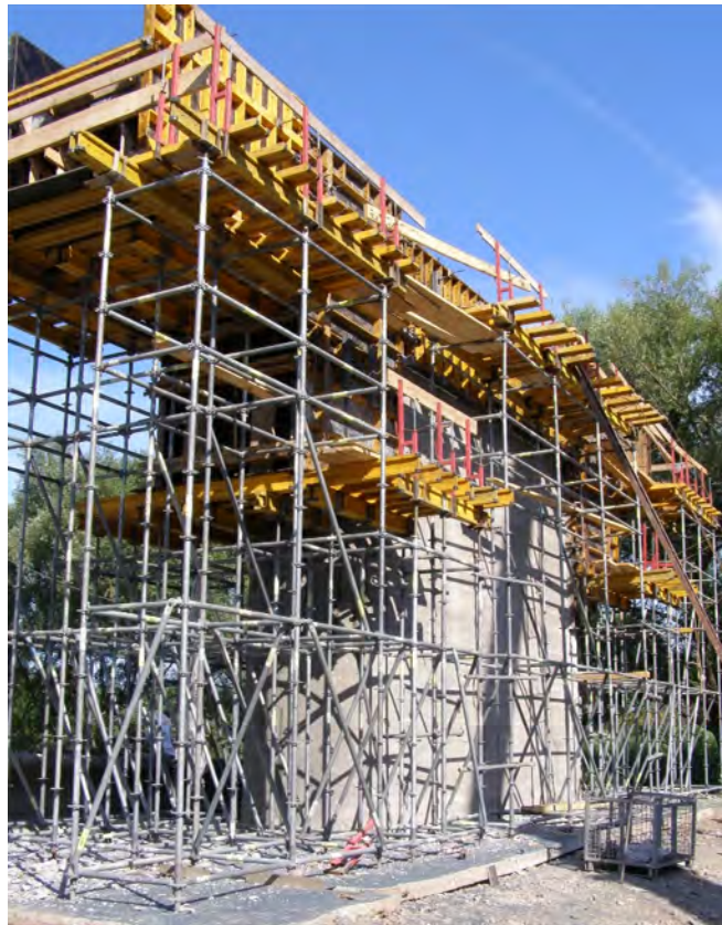
Figure 1 – Example of a high-rise formwork system for the reconstruction of a bridge supports. Concreting works were carried out using SCC
