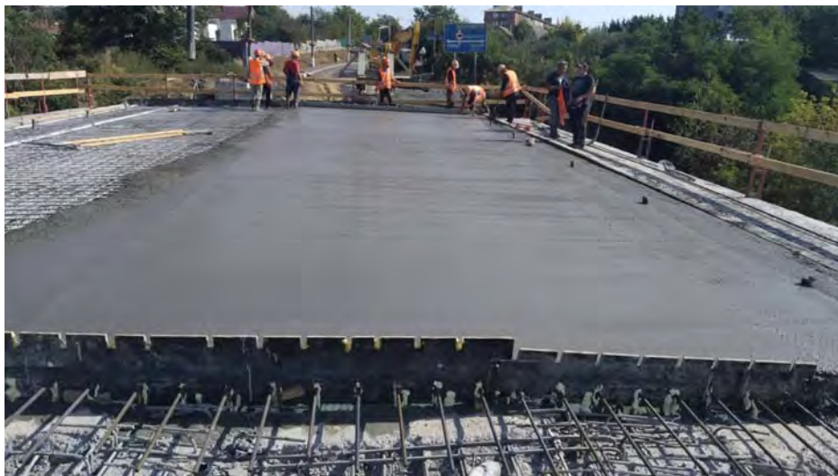
Figure 2 – Concreting of the overhead slab of the girder structure using SCC based on superplasticizer
