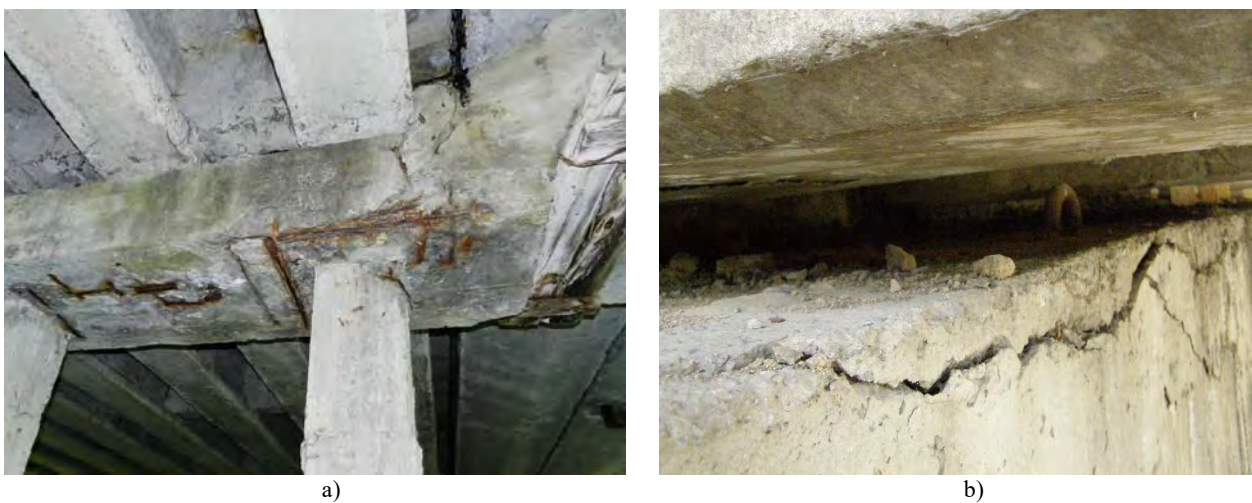
Figure 3 – Typical defects and damage to the crossbars: a – destruction of the protective layer of concrete with exposure and corrosion of reinforcement, b – wide longitudinal cracks of the protective layer of concrete in the stretched zone, which indicate defects in the working reinforcement.
